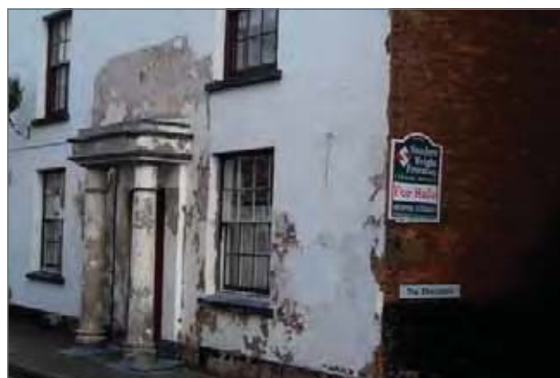
Need for maintenance and repairs to retain components
